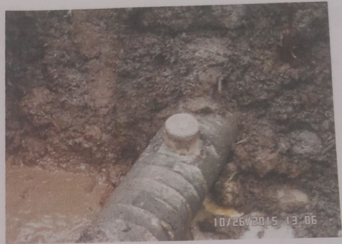
BUNKERING POINT SHOWN
